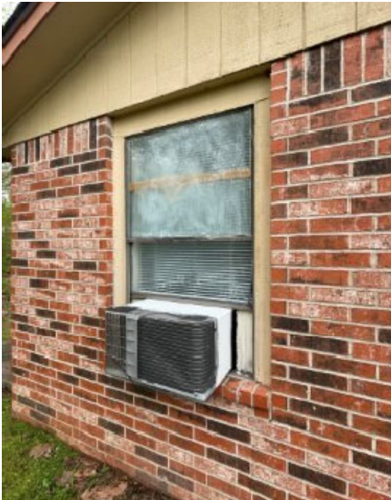
Office window unit
